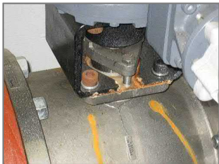
FCV Actuator Bolts Corrosion
