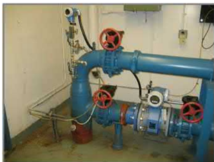
Paint Fill Piping
