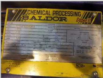
Motor Nameplate: Not Inverter Duty
