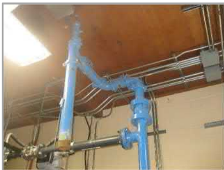
Corrosion & Open-ended Pipe
