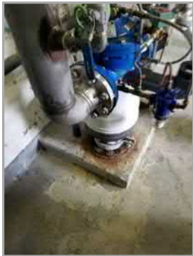
Bad Welding, PRV and Level
