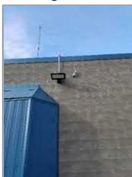
Exterior LED Lighting
