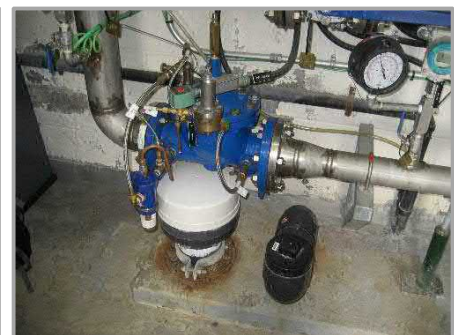
Level Transmitter Access Blocked
