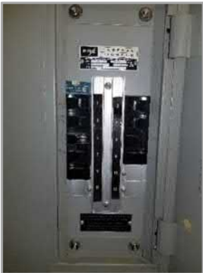
Rusting Distribution Panel
