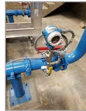
PIT with Tiny Pressure Gauge
