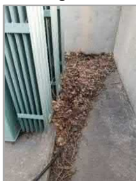
Debris Behind Transformer
