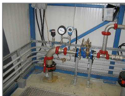
Valves and Piping
