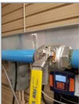
Rusting Isolation Valves
