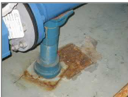
Pipe Support Rust
