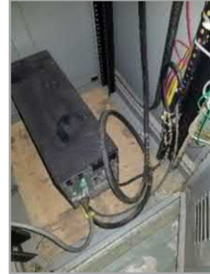
UPS Mud Covered
