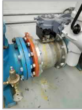
Flow Control Valve; Rust Stains
