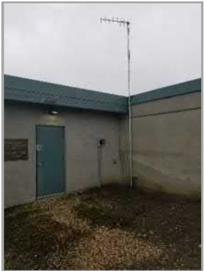
Antenna and Power Meter
