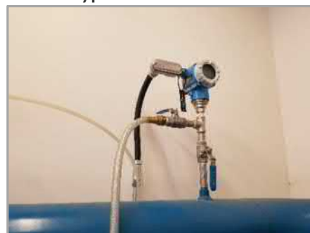
Tap Before Pressure Transmitter
