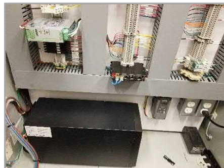
UPS and Single Power Supply
