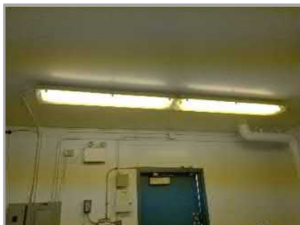
Lighting and No Exit Light
