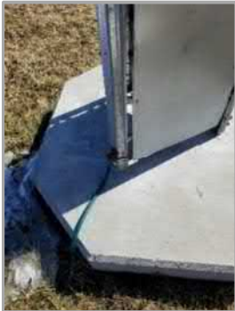
Radio Tower Ground
