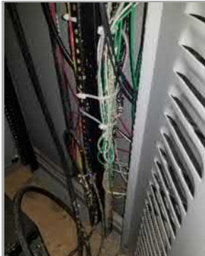
Mud Covered Wiring
