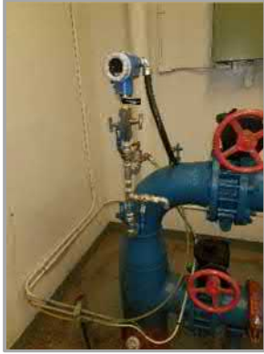
Inlet PIT and Analyser Feed
