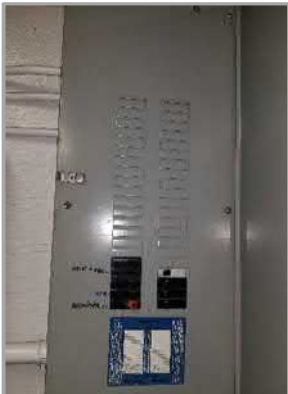
Oversized Distribution Panel
