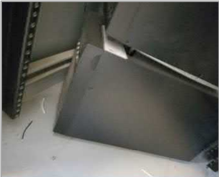
UPS with Battery Extension Pack
