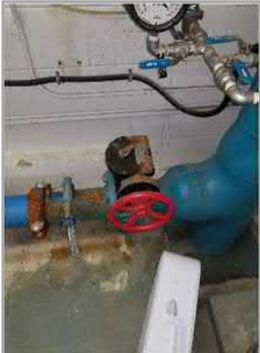
Rusted Piping and Valve
