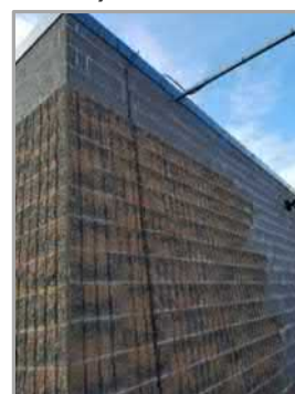
Lightning Down Conductor
