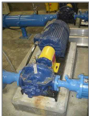
Head Bolts – Superficial Rust
