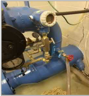
Inlet PIT and Analyser Feed
