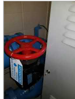
Valve Blocks Rear Cabinet Door
