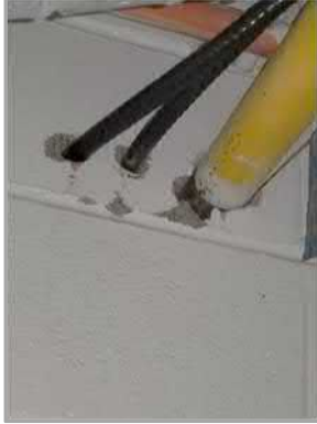
Penetrations Not Sealed
