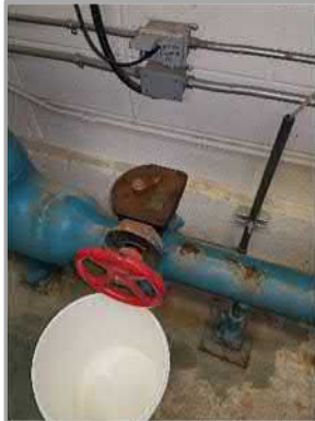
Rusted Valving and Piping
