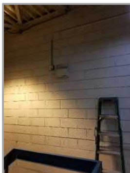
Interior Emergency Lighting
