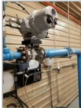
Flow Valve; Rusting
