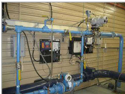
Corrosion on Fittings
