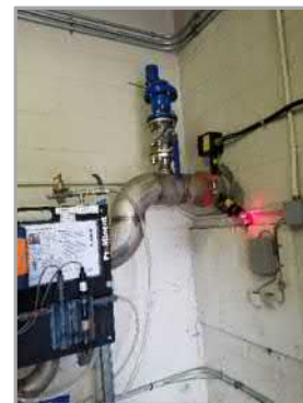
Incoming Line, ARV & Heat Trace
