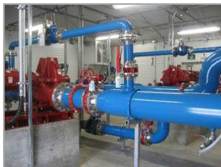
Equipment and Piping
