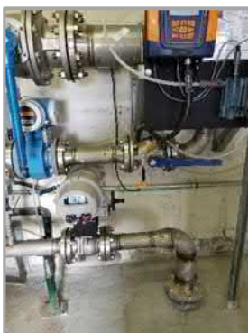
CL 2 Analyser and Piping
