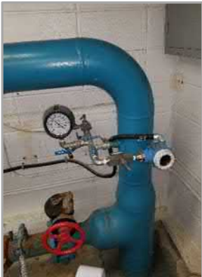
Inlet PIT and Analyser Feed
