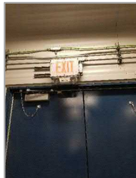
Exit Sign with Lights
