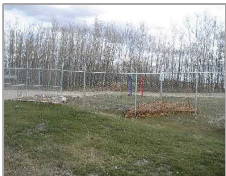
Gap Under Fence
