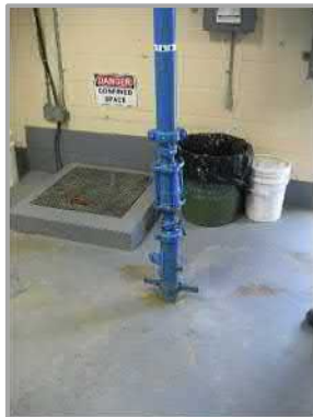
Pipe Stability Concerns
