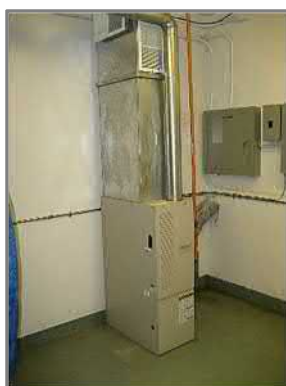
Force Air Furnace
