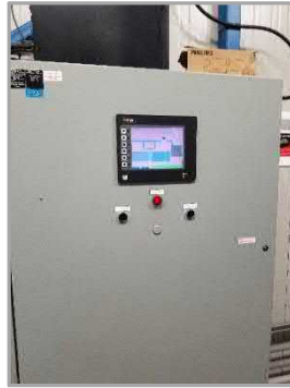
PLC Cabinet with HMI
