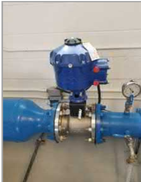
Flow Control Valve
