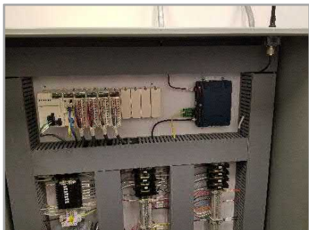
PLC Rack and Radio
