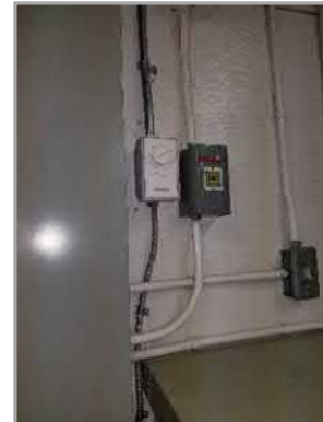
Power Fail Relay
