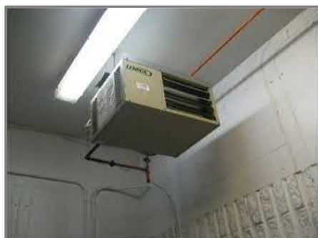
Ceiling Mounted Air Handling Unit
