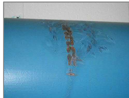
Pipe Surface Scuffing
