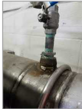
Corroding NPT Weld
