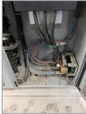
VFD interior; dusty
