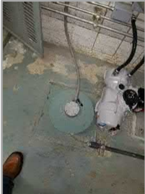
LIT Access - Is Water Return Sealed?
