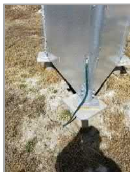
Radio Tower Ground
