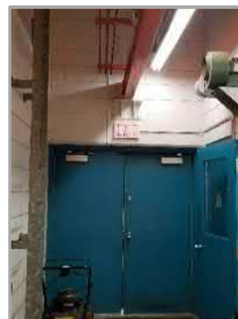
Main Entrance: No Emerg. Lighting
