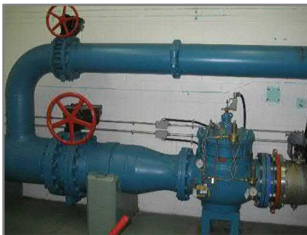
PSV and Piping - Condition
