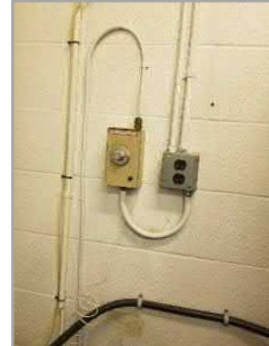
Heat Trace Controller
