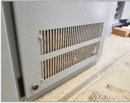
VFD Intake Filter; Plugged
