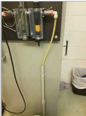
Drain Line Needs Air Gap
